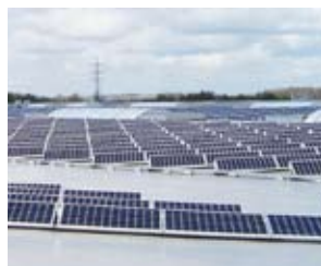
Our new Aalst warehouse boasts solar panels
