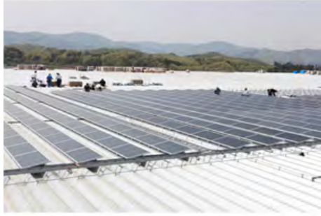
The building's megasolar power generation facility (top)
