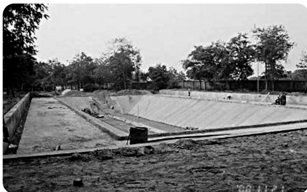
Controlled type landfill facility installed on plant grounds
