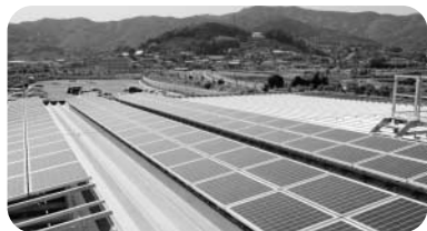
Solar cell panels installed on the roof of the plant
