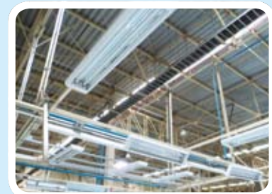
Fluorescent lights have been replaced with energy-efficient 25W bulbs.
