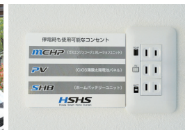
During an emergency, the gas cogeneration unit, solar panels, and home battery unit generate and supply electricity. After their specifications have been determined, these devices will connect seamlessly to all electrical outlets to monitor and balance supply and demand.
