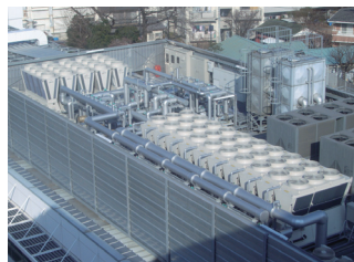
Heat source equipment (15 modular chillers)
