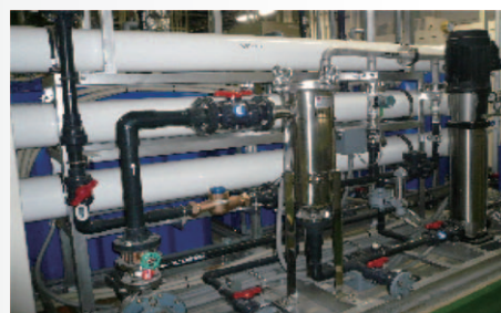
RO membrane - based wastewater treatment system
