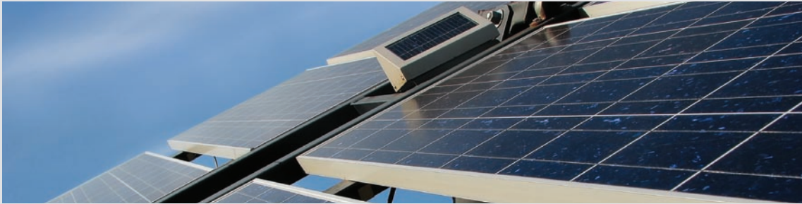
South Marston Solar Park – 21.300 panels cover 13 ha of land generating 4.2 to 4.6 GWh of electricity per annum. A percentage of the solar panels are manufactured by Honda's own Soltec Company.
