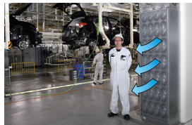
Air diffuser installed on the lower end of a pillar inside the factory
