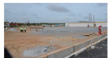
Rain-water harvesting system reduces ground-water use by 20,000 tons per year
