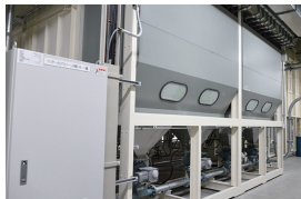
Dry spray booth installed for bumper coating
