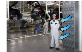
Air diffuser installed on the lower end of a pillar inside the factory
