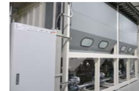
Dry spray booth installed for bumper coating
