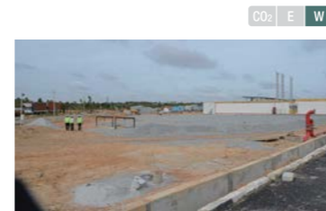
Rain-water harvesting system reduces ground-water use by 20,000 tons per year
